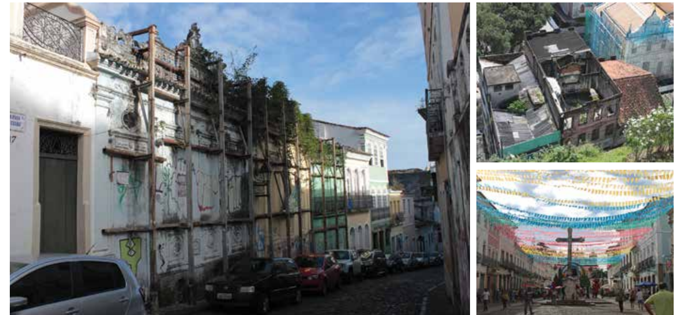
Clockwise: Abandoned building on Ladeira do Carmo. Metal structures supporting old buildings are commonly seen throughout the surrounding streets of Pelourinho. Abandoned buildings without roofs are common in the deteriorated Cidade Baixa. Largo do Cruzeiro do São Francisco in the heart of Pelourinho on an early winter afternoon.
